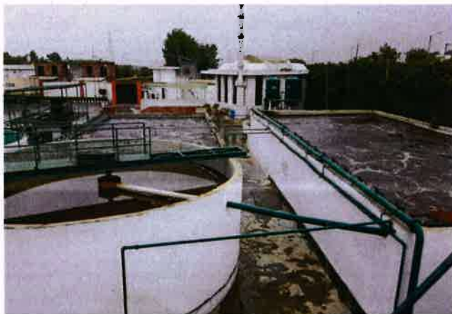
Effluent treatment plant, installed capacity 1000kld based on two stage activated sludge process , WITH DAF.
