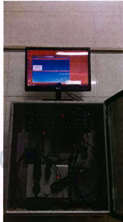
Online automatic effluent monitoring equipment installed at the end of ETP
